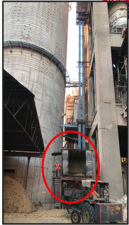
Enhance capacity of Line-3 Rice Husk system (5 TPH to 15 TPH)
