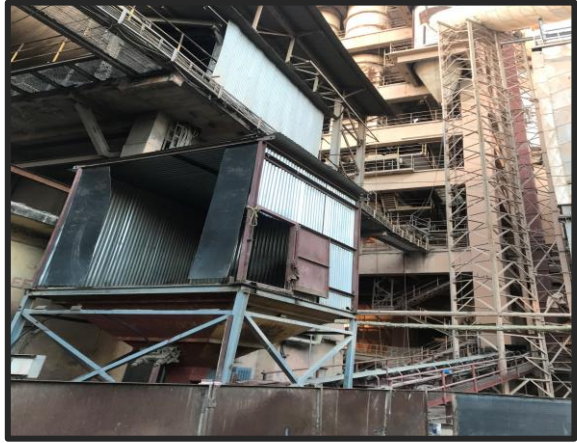
Line -3's 5 TPH Rice husk feeding system installed in Line-2
