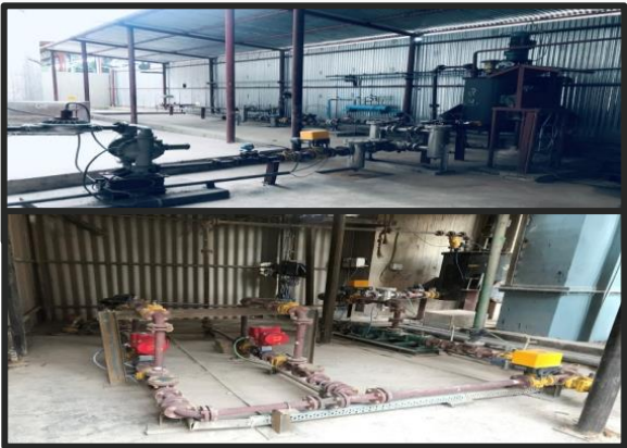
LAFR System in Line-3
